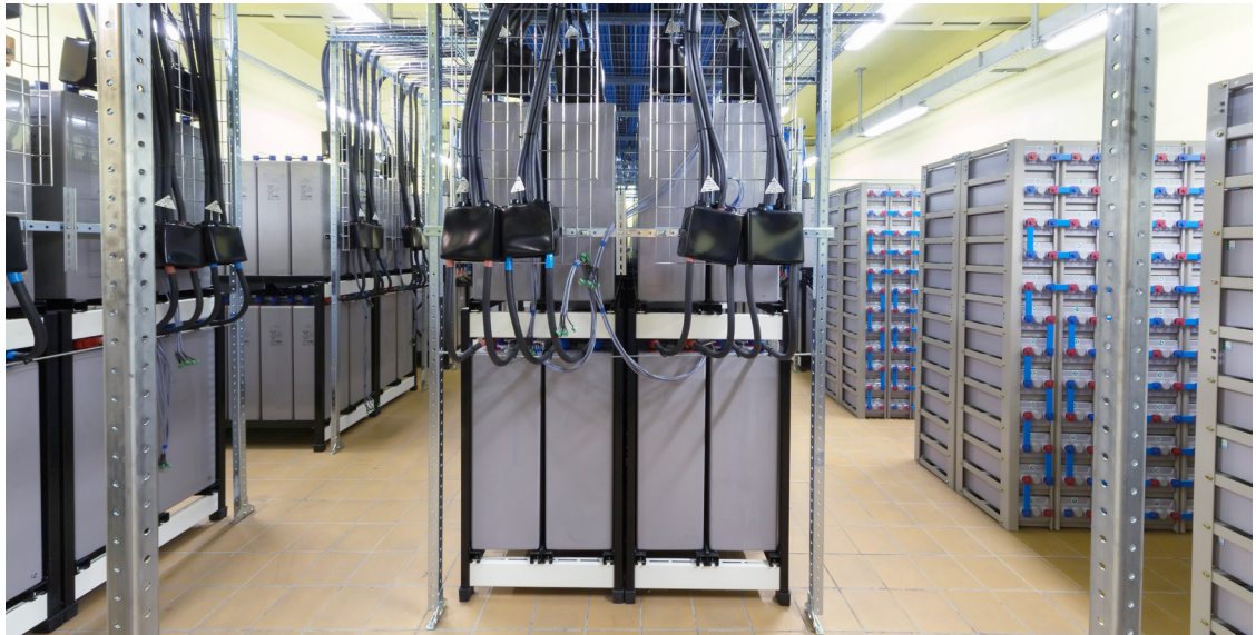
Batteries are an important source of malfunctions in many data centers due to lack of maintenance.
